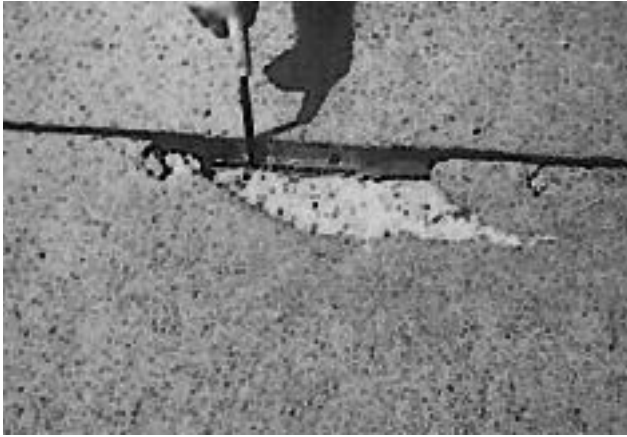
Figure 1. Transverse joint spalling.
