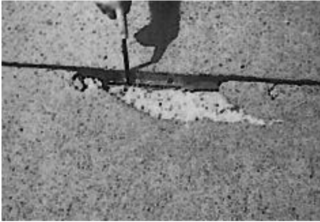
Figure 1. Transverse joint spalling.
